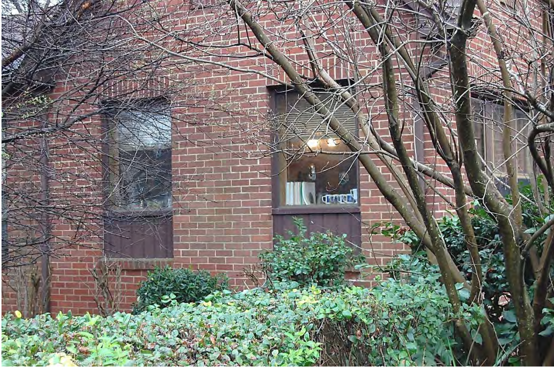
John and Roselie Stewart House, Side (West) Elevation, Replacement Windows.
