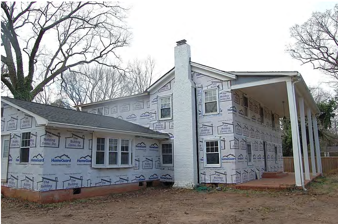
James B. and Malissa N. Williamson House, Side (East) Elevation and Wing, Looking Southwest.
