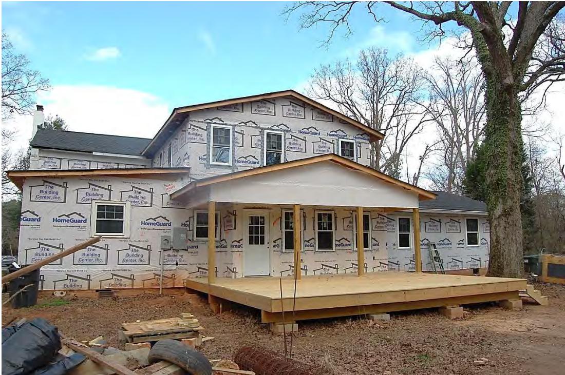
James B. and Malissa N. Williamson House, Rear (South) Elevation, Looking North.
