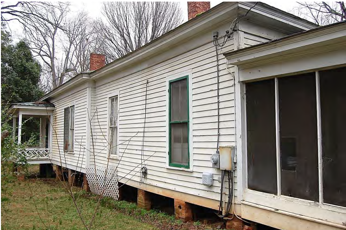
McLaughlin-Bost House, Rear Ell and Rear Wing, Side (West) Elevations, Looking East.
