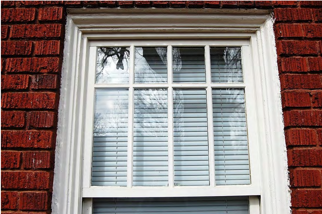
Renfrow-Lemmond House, Side (East) Elevation, Replacement Window.
