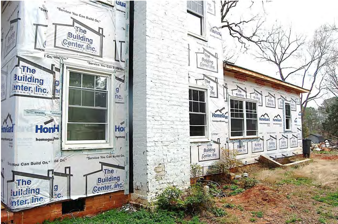
James B. and Malissa N. Williamson House, Side (West) Elevation, Looking Southeast.
