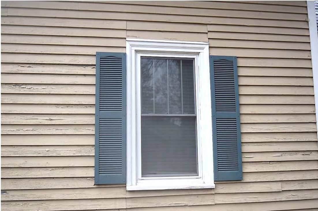
Sidney J. and Shelby W. Hooks House, Side (North) Elevation, Replacement Window.
